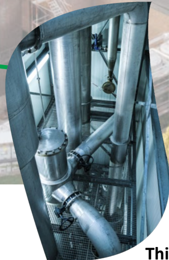
Spray dryer room
